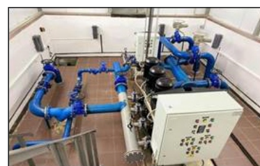
Pumping station of Makinsk CWM (Akmola province)
