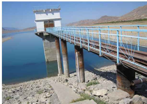
Tower outlet at a dam in Kyrgyzstan
