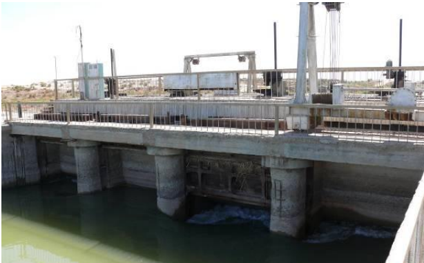
A regulator at Khanhovuz canal in need of renovation
