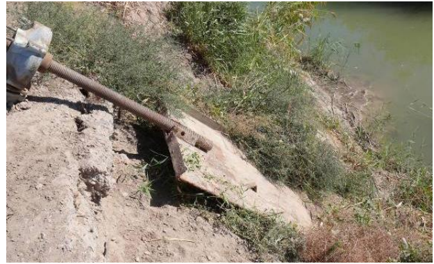
A deteriorated section of the irrigation canal
