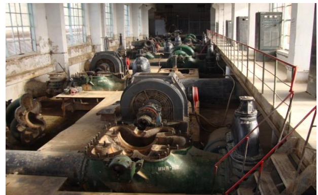
A cascade of five pump stations supplied irrigation water to lands around Garauti
