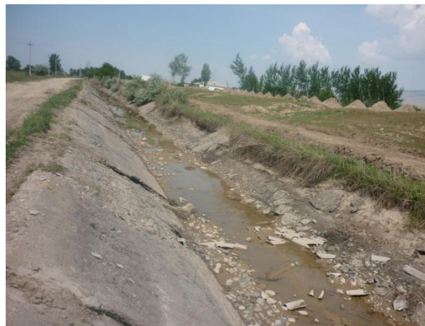
Bad Bad irrigation canal before rehabilitation
