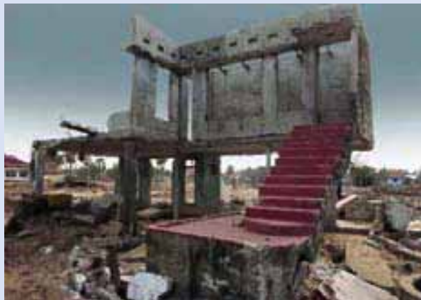
Mullaitivu, a town in Northeastern Sri Lanka ravaged by the tsunami of 26 December 2004
