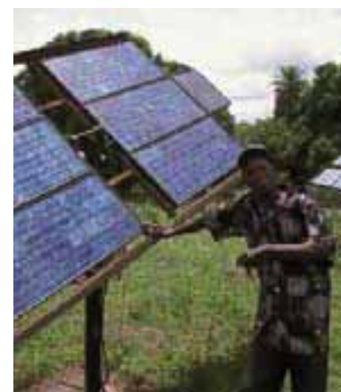
This solar voltaic panel's energy is used to pump water, Kabekel village, Gambia
