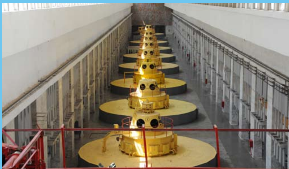
Visit to Nurek HPS power room (on the lower picture).
