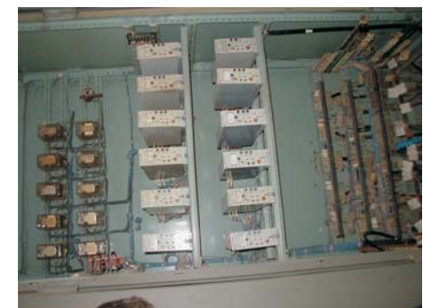
Fig. 3. Cupboard with transformers
