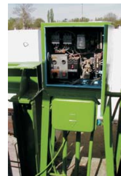
Fig. 2. Cupboard for gates local control
