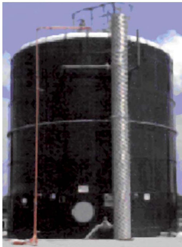
Fig. 6. Biogas Facility for Combustible Methane Production
