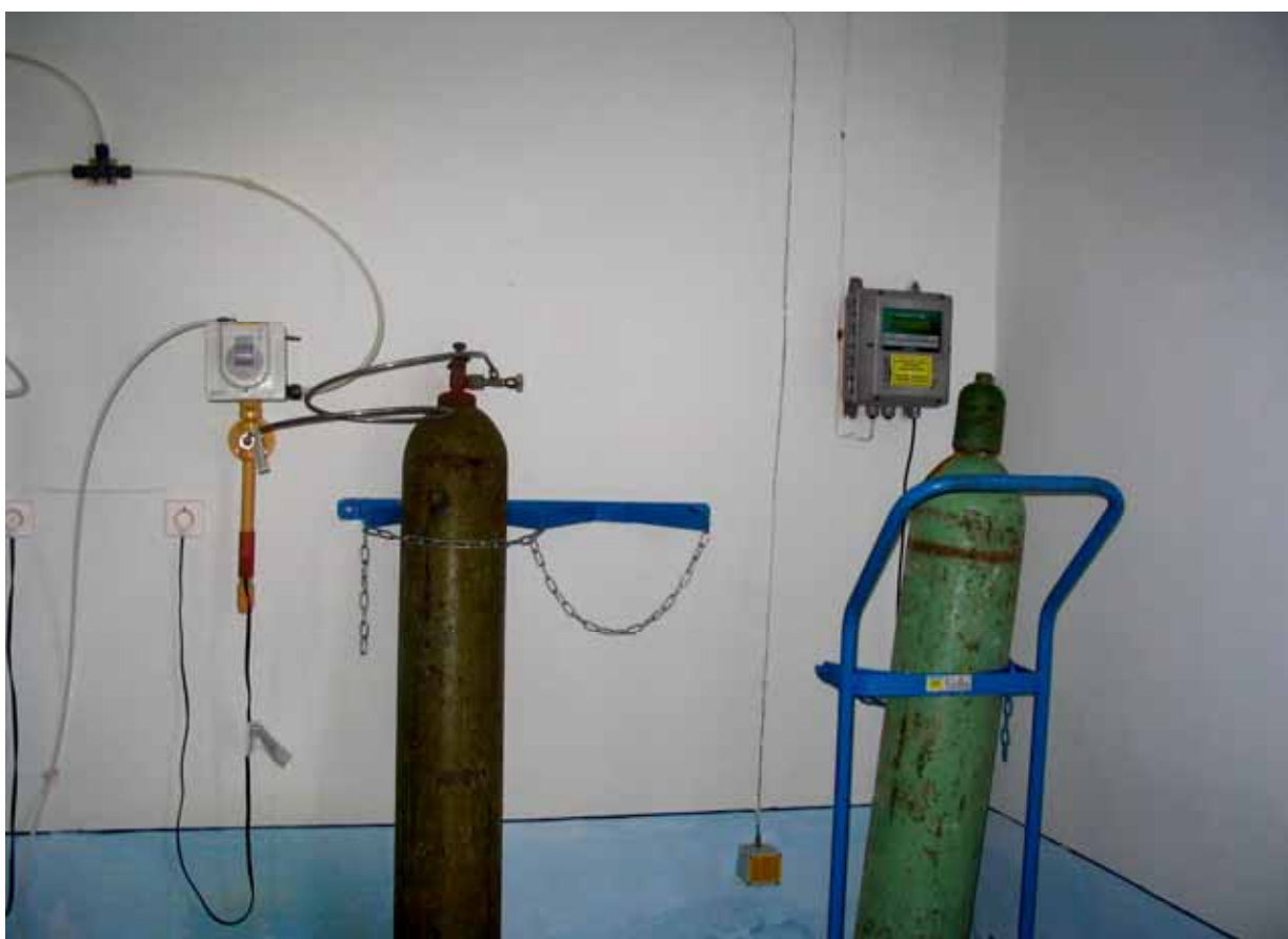
The tap water disinfection with liquid chlorine.
