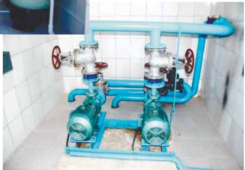
Water pumping units
