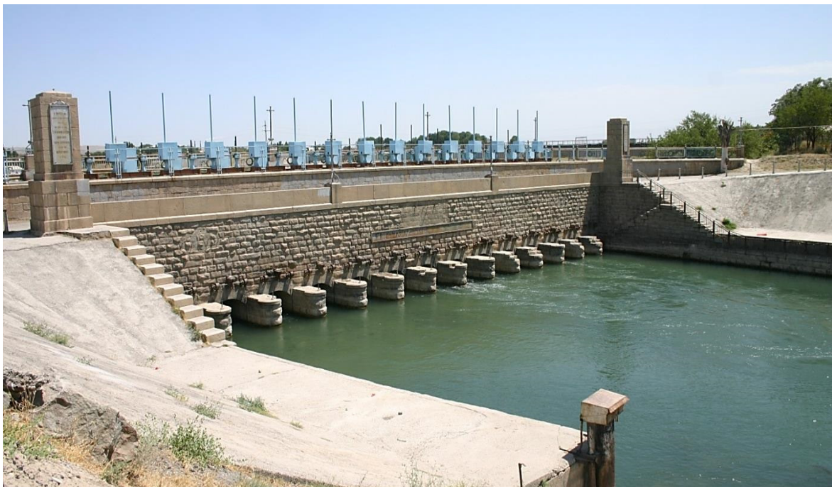
Figure 4. The head structure at the Dustlik (“Friendship”) canal (in the Soviet years, the Kirov Canal. It starts from the derivation channel of the Farhad hydroelectric station.
