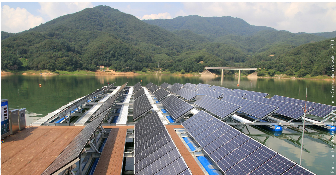
Renewable energy generated by these floating photovoltaic systems reduces carbon emissions at Hapcheon Dam in Republic of Korea.
