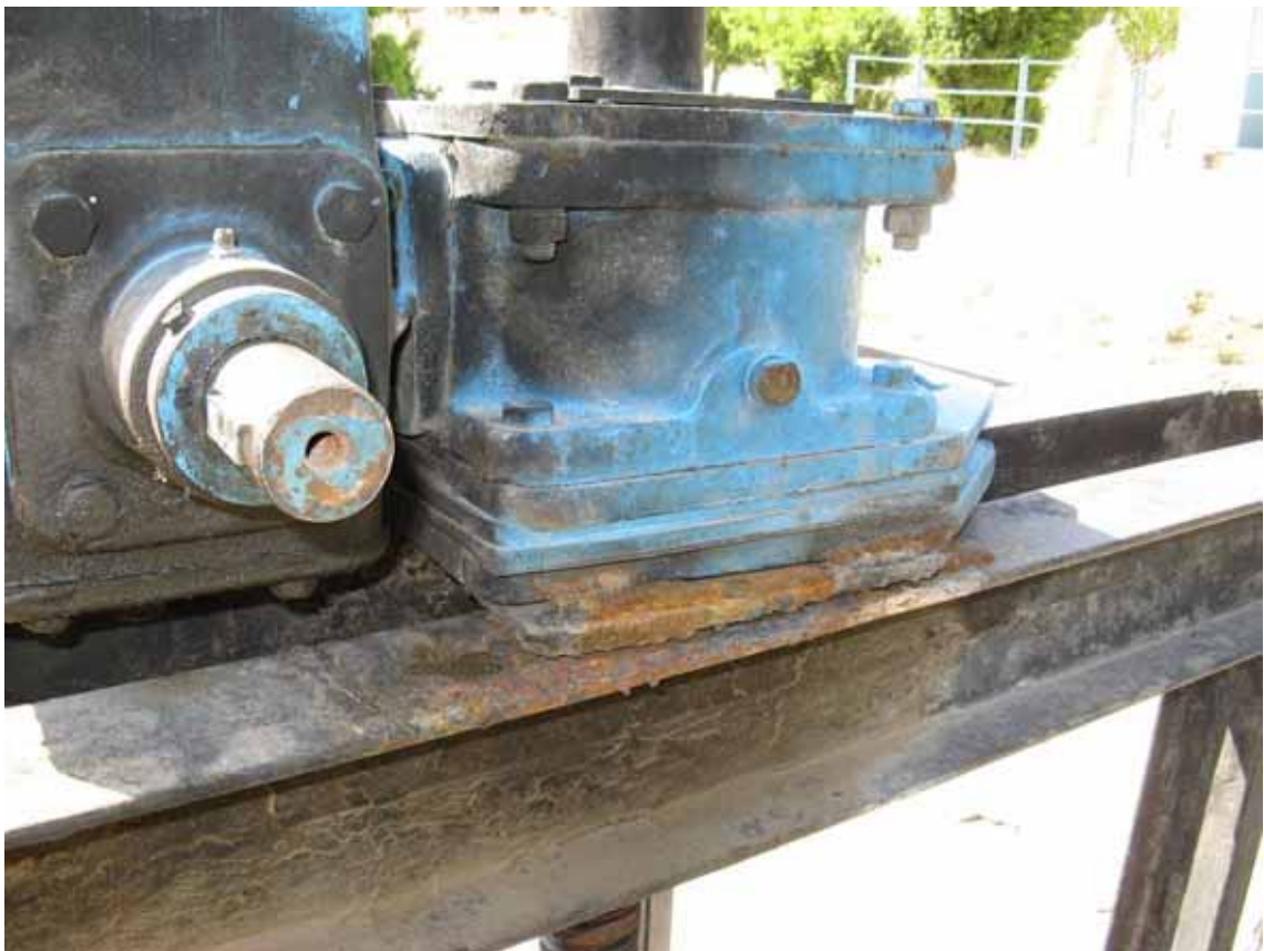
Broken reducer welding at point 2
