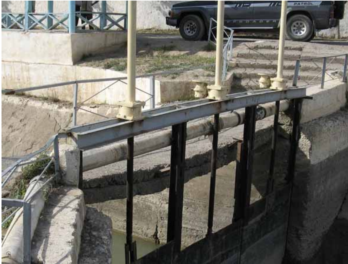
Missing reducers at point 5
