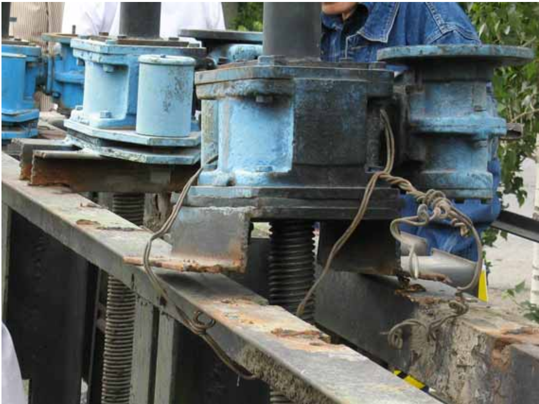
Broken reducer support at point 6
