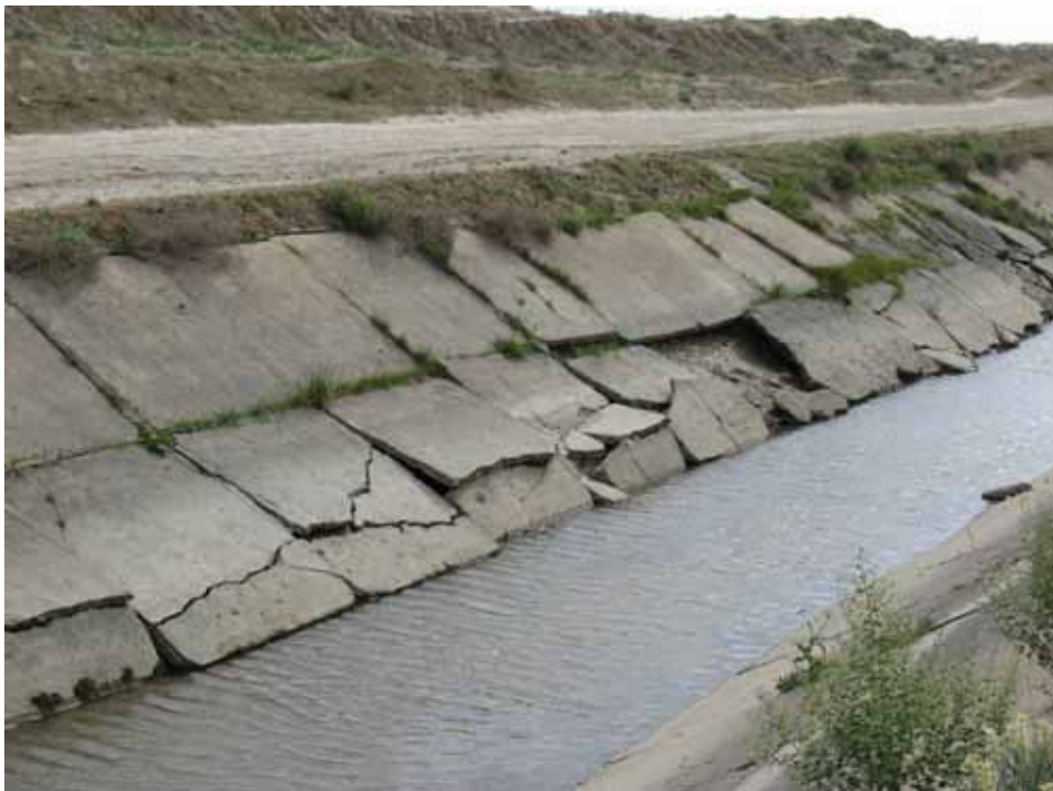
Damaged canal lining at point 4
