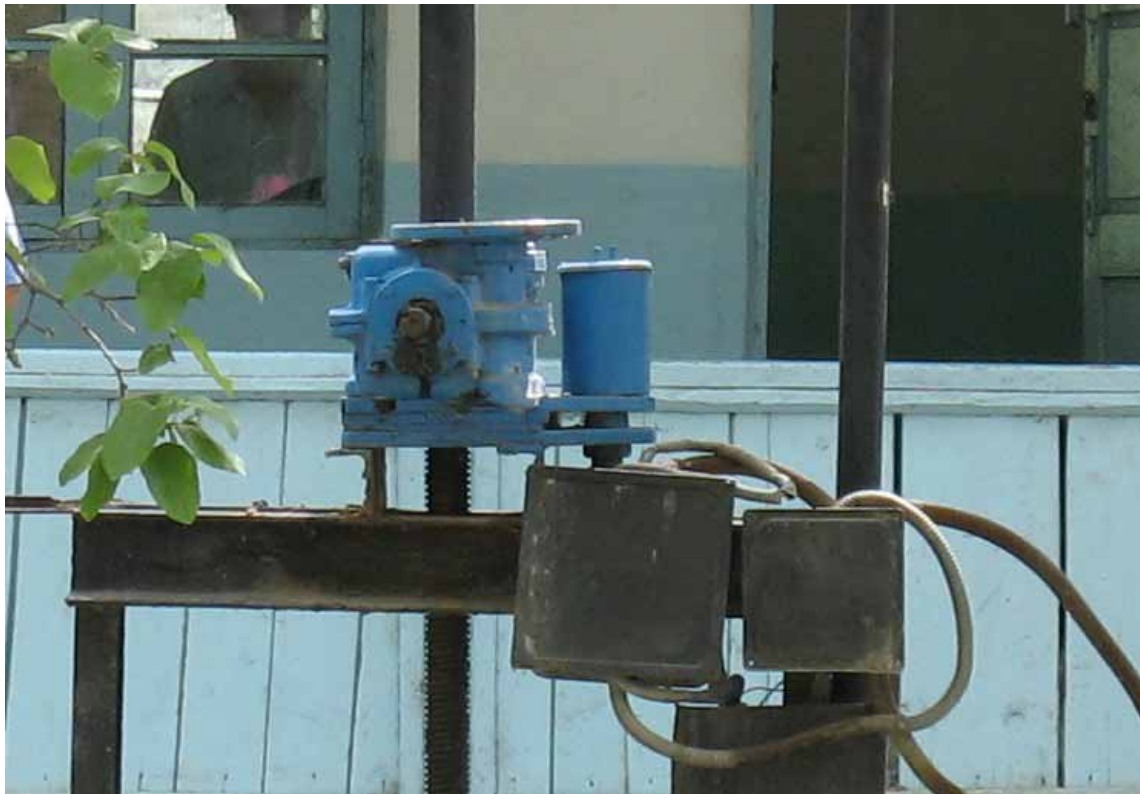
Non-horizontal reducer at point 6
