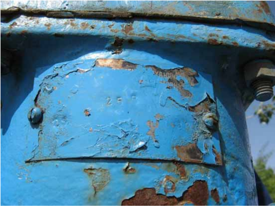
Bad condition of reducer at point 6
