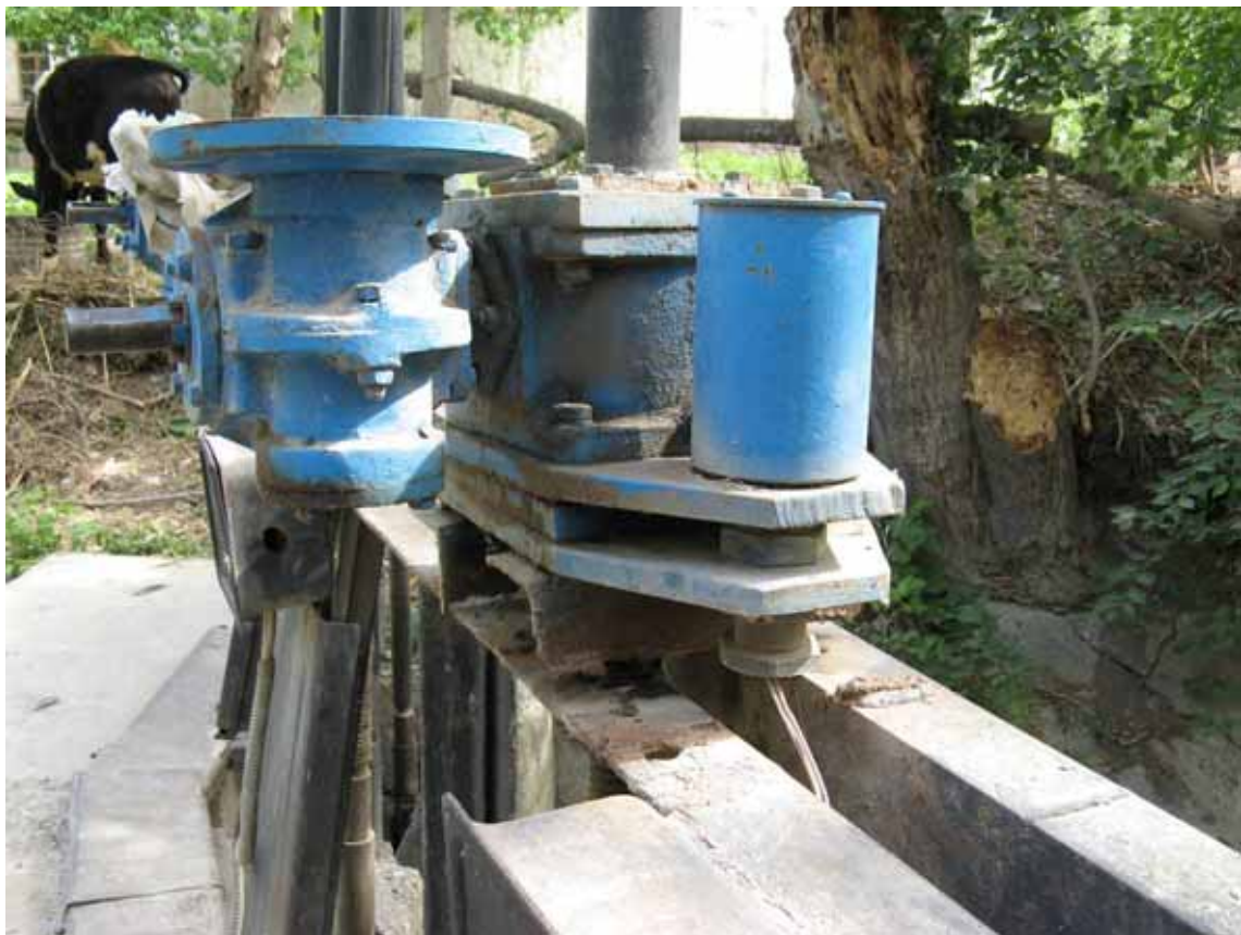
Broken reducer support at point 6
