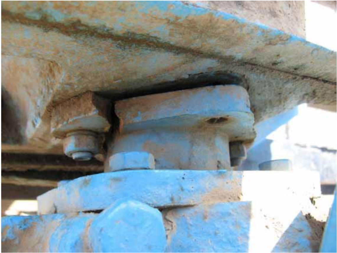
Broken reducer casing at point 3
