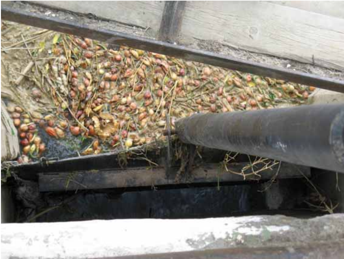
Bent gate at point 6
