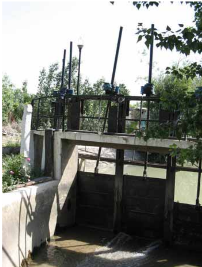
Broken reducer support at point 6
