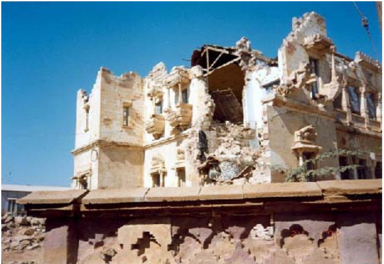
Figure 4.3.1 Devastation of a building in an urban area during the Bhuj (India) earthquake of 26 January 2001. The earthquake caused complete failure of basic amenities, including the water supply system
