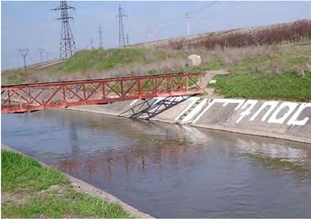
Gauging station on the main canal (SFMC)
