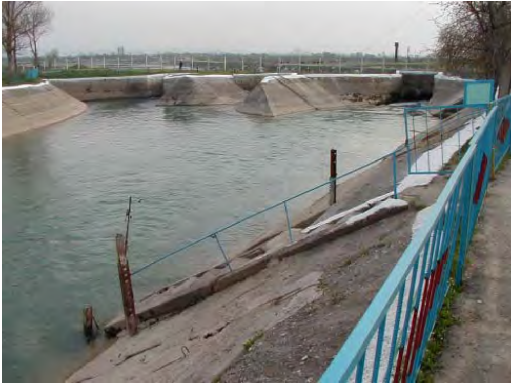
SFMC (hydraulic site)
