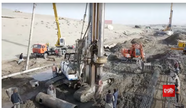
Figure 1. Deserted areas in the north of Afghanistan at the very beginning of Qoshtepa Canal construction.
