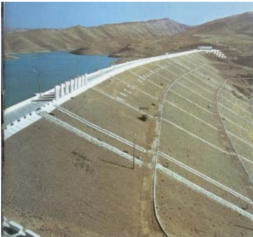
Figure 17. Pachkamar Dam on the Guzardarya River, Uzbekistan (dam's height – 71m; water storage volume – 260 mln. m 3 )
