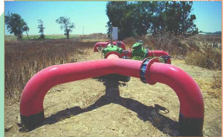
Mix junction using effluent and saline water.
